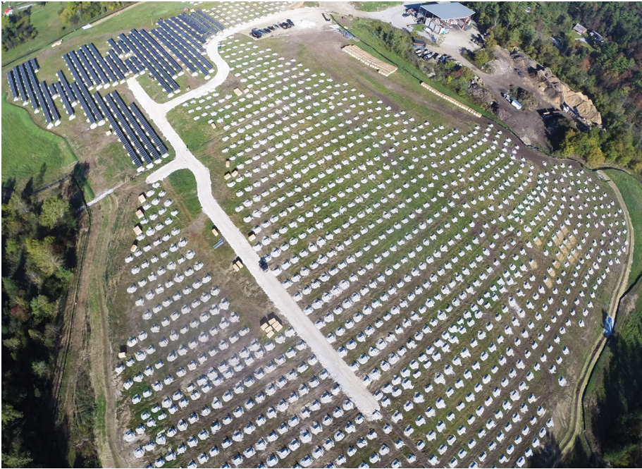
The Stafford Hill solar project also includes 4 MW of battery storage. Vermont's governor attended the groundbreaking ceremony. Photo courtesy of Green Mountain Power
